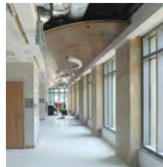
A look down the first-floor hallway that will connect the new wing to the old building near the current site of PU's Coffee.
