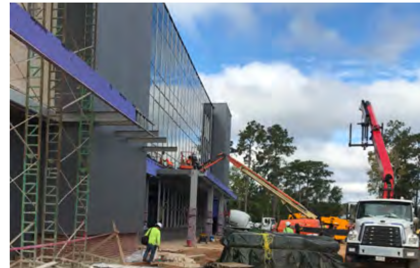
A new cancer center goes up near the intersection of Highway 21 and Interstate 12 in Covington. The center, a joint project of St. Tammany Health System and Ochsner Health, is expected to accept its first patient in summer 2021. (Photos courtesy Ochsner Health)
